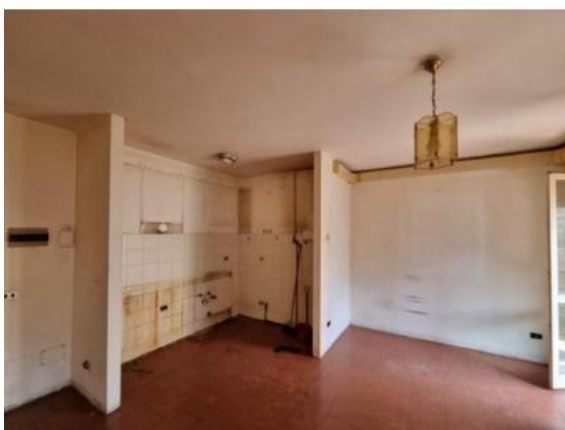
Figure 1 - Condition of the flat prior to the refurbishment work carried out by MM.
